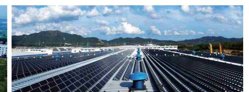
Solar panels arrays
